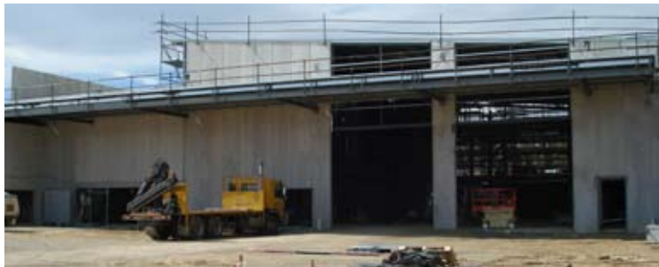
A view from what will be the carpark of the new Mitchell store showing the entry to the warehouse on the right and to the Southern Plumbing Plus trade area on the left.
