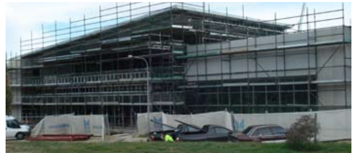
Scaffolding erected to install the glass on the Southern Innovations showroom in Flemington Road Mitchell.
